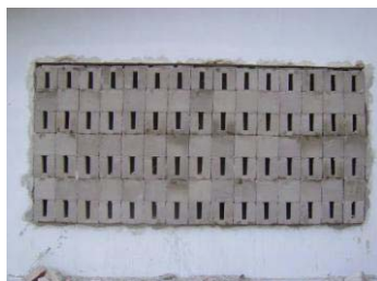
Figure 19: Photo of the block type box (open - external view)
