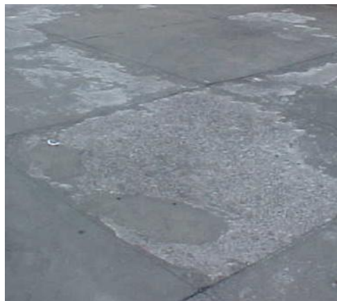
Figure 6. 1 – Abrasion wearing on the surface of a concrete industrial floor.
