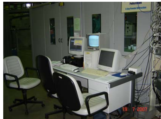
(b) painel de controle
