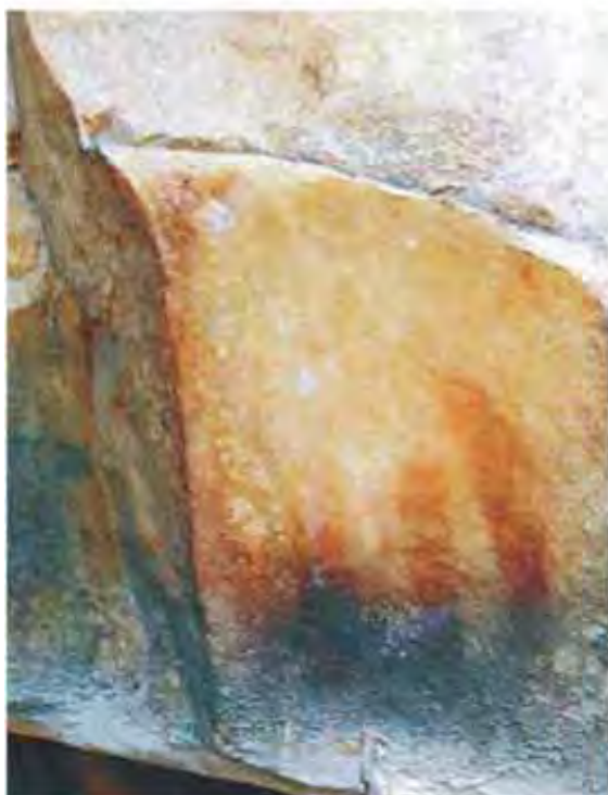
Escarpa da Silvaneide - BOME-15 Painel 12. RT-16
