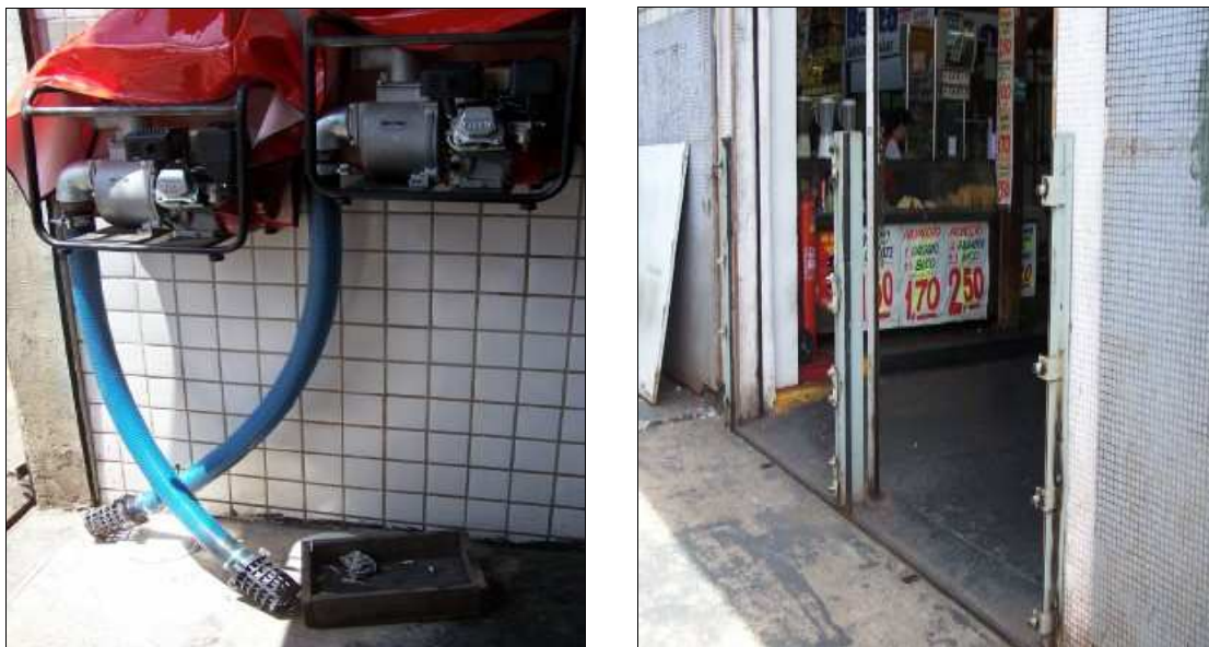
Figura 45. As bombas de água e as comportas do Mercado Municipal (Foto do autor, 10/01/2006).
