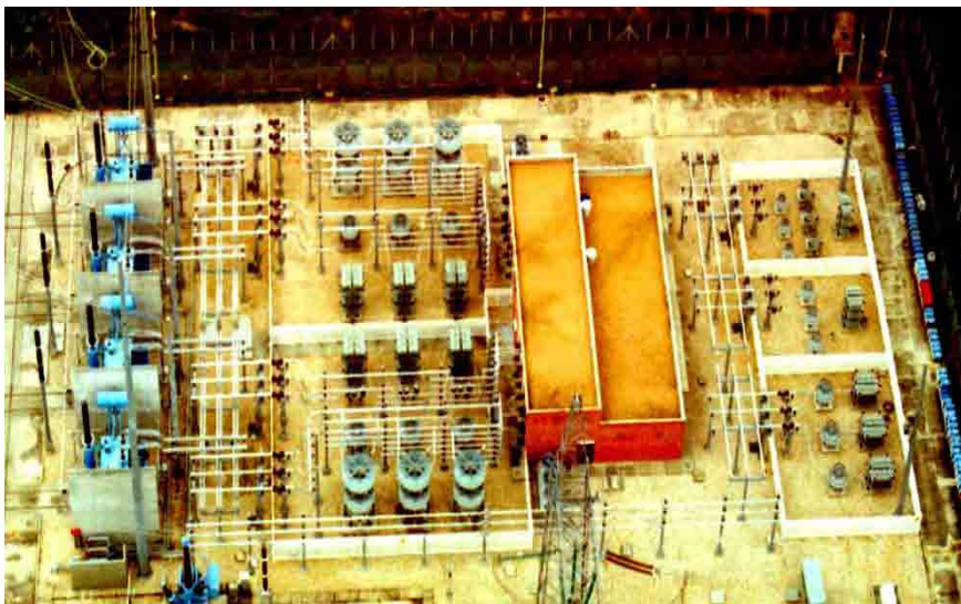
Fig. A.8: Plataforma SVC China – 500kv, 250 MVar-cap. / 150 MVar-Ind.
